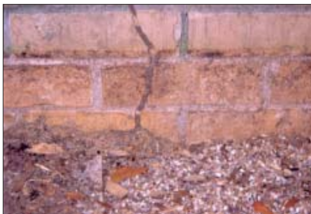
Figure 4a. Termite shelter tubes on foundation wall.
