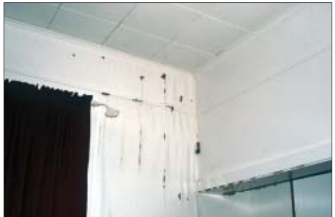
Figure 12. Shelter tubes on interior walls.
