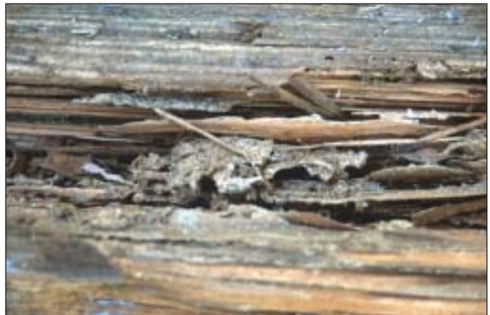
Figure 10. Termite damage in wood.
